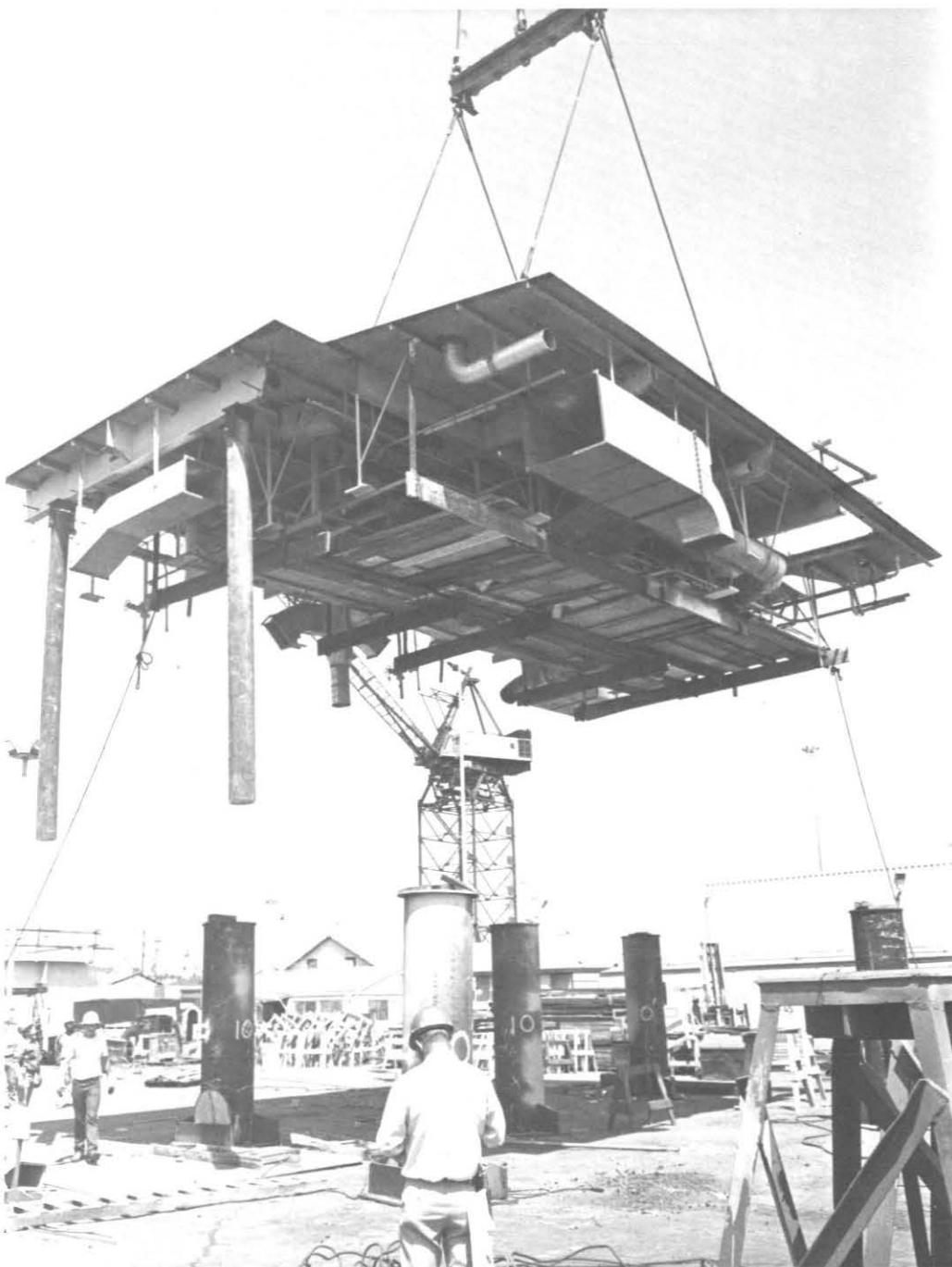
A 40-foot flat at the beginning of its trip from the building ways to its location on Mercy. This unit will rest directly over diesel generators in the auxiliary machinery room. Note the ducting and piping already in place.
